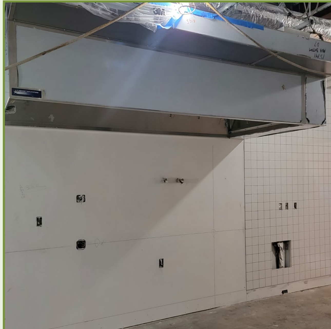
2 nd Floor - Catering Kitchen
